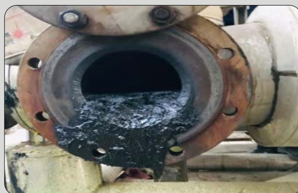
Soft and sooty material in rundown lines - 2.12.21
