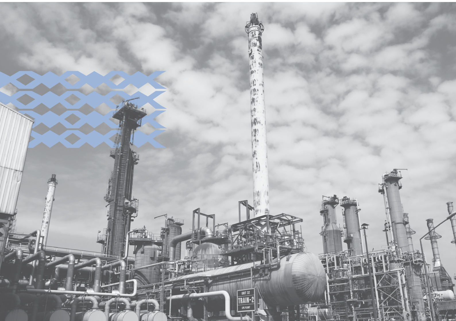
Mina Al-Ahmadi Refinery Gas Liquefaction Plant
