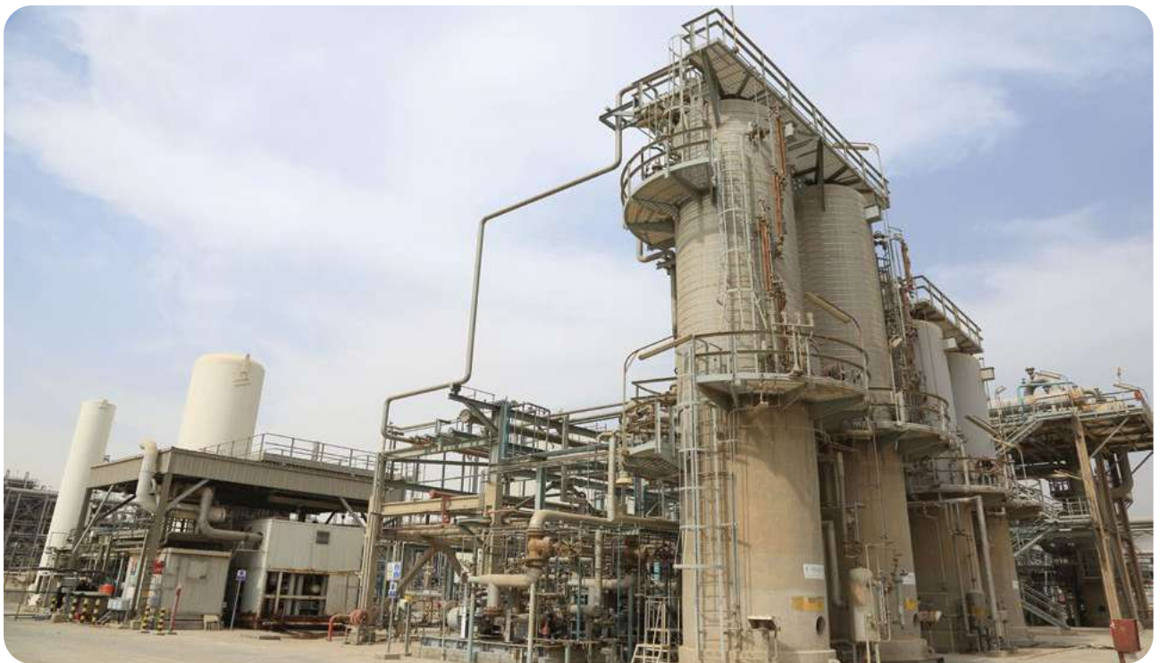
Flare Gas Recovery Unit at Mina Al-Ahmadi Refinery
