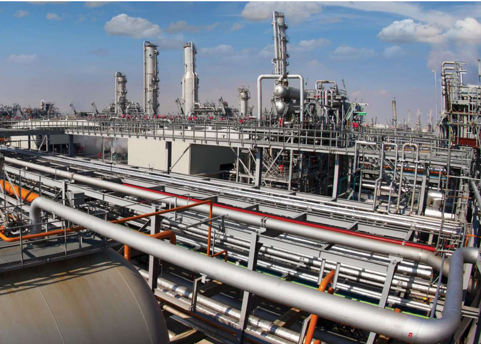
Fourth Liquefied Petroleum Gas Train
