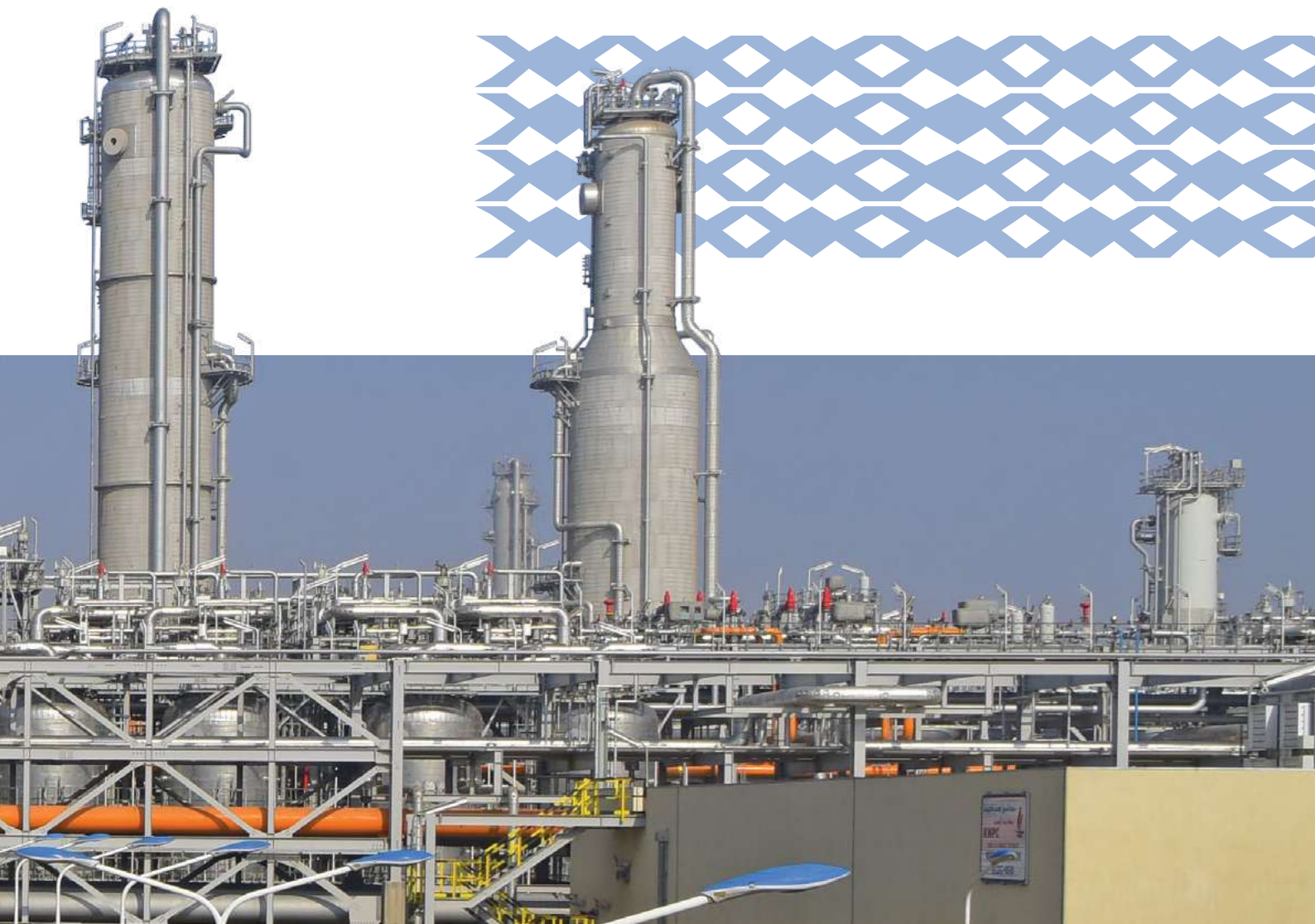
The 5th LPG Train at Gas Liquefaction Plant
